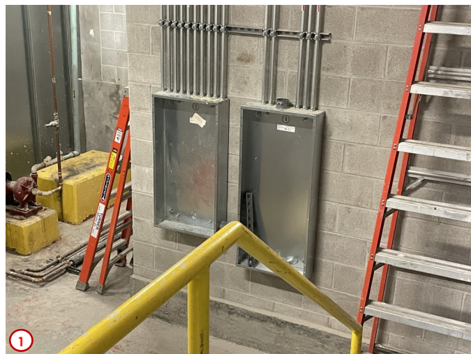
Photo #1 shows the future home of the building power and lighting panels in the Mechanical Room in the Basement. Thanks to the construction of the new Janitorial Closet the bare wall was able to be used to house these new panels where they will be both accessible and centrally located for maintenance reasons.
