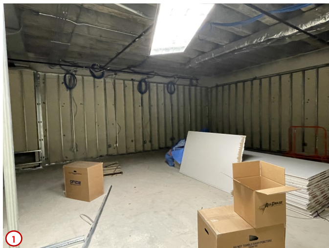
Photo #1 was taken in the old distance learning classroom in the north-west corner of the basement. This space is designated as a computer lab, however first all the walls are receiving metal furring channels and a layer of wallboard to create a smooth finish. This space like the rest of the basement will also receive new suspended acoustical tile ceilings and LED lighting.
