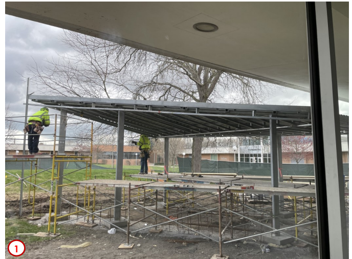
Photo #1 shows the contractors at the beginning of the week starting the rough framing for the new east entrance canopy. The underside of the canopy will be finished so that it appears similar to that of the building's soffit. Then the face will receive a light-gauge metal flashing, and then the roof a fully-adhered membrane roof. Once the building roof replacement is complete and the contractor off site then the work on the new west entrance canopy will begin.
