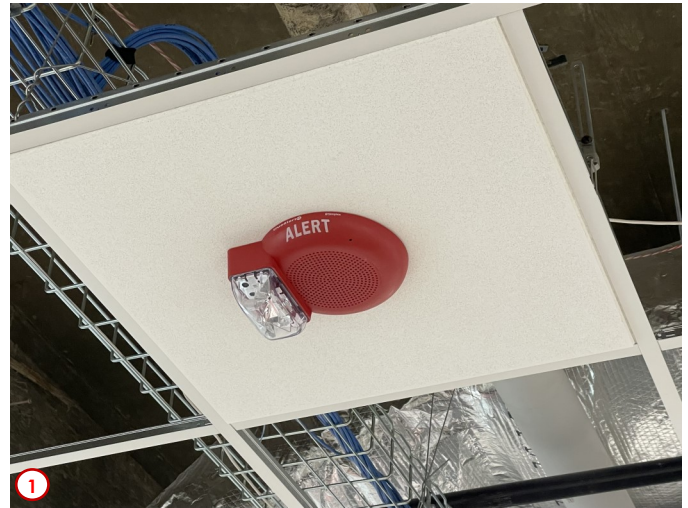
Photo #1 highlights one of the many new warning strobes and annunciators that are part of the new building-wide safety systems. With all of these in place and the proper inspections have taken place this week the contractors will begin to “pad” out the rest of the ceiling tiles to finish the ceilings on the 2nd floor.
