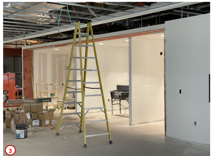
Photo #4 shows one of the many areas on the first floor where some of the necessary preparations are being made to the existing slab to receive the future floor finishes. Here you can see where some thin set concrete has been used to help create a smooth transition of an area where there was a difference in flooring heights. This is so that once the new carpet planks are installed there will be no unintentional trip hazards for building occupants.
