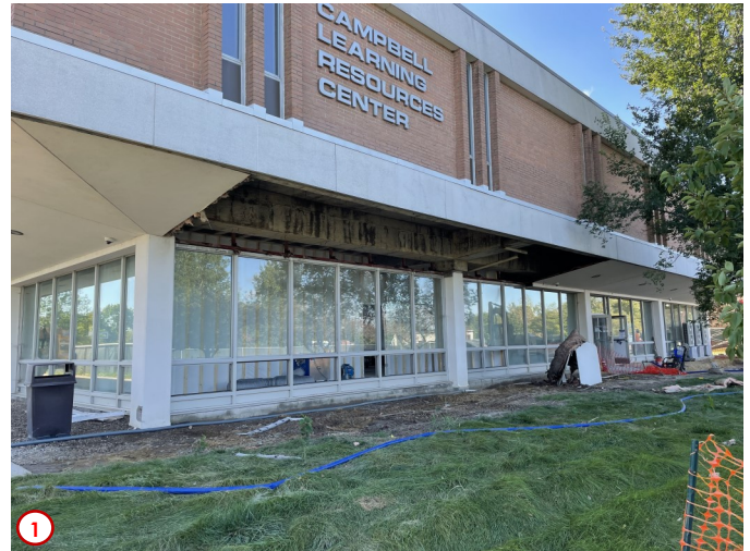
Photo #1 was taken outside the exterior northwest corner of the CLRC, and shows the completed demolition to the existing soffit that will allow the new addition to start in this area. This addition will hold three of the five new huddle rooms planned for the Library when all of the building renovations are complete.
