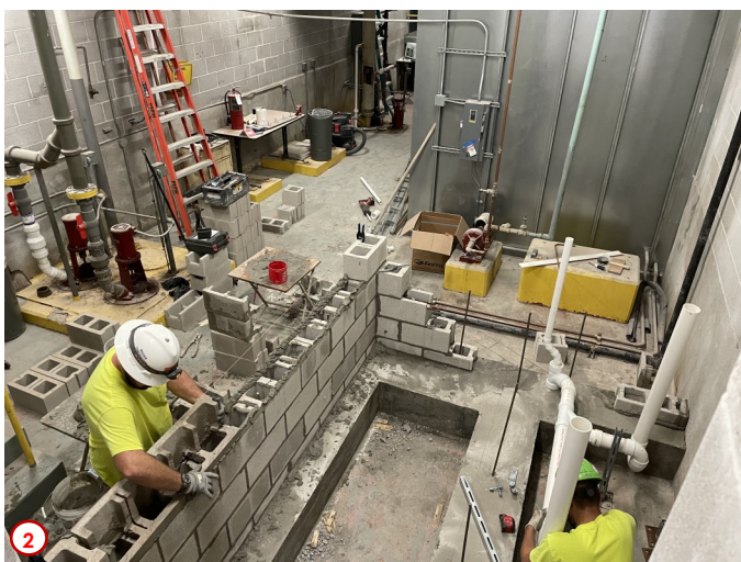
Photo #3 is of the same area as Photo #2 but taken later in the week and from a different viewpoint. Here you can see the walls are finished up to a certain point and the metal decking has been installed. Next week the new concrete floor slab will be placed on the metal decking so that the floor level in the new janitor's closet will match in elevation that of the adjacent corridor in the basement. Then once the slab is cured enough the masonry contractors will come back in and finish laying the remaining portions of the block walls up to the floor deck above thus separating this new space from the rest of the existing mechanical room.
