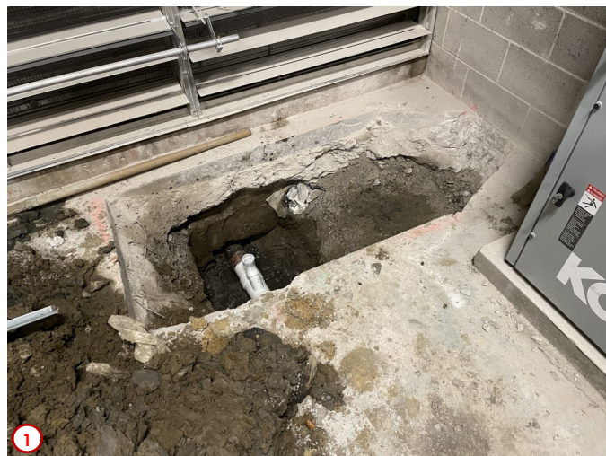
Photo #1 was taken in the existing basement electrical room. Here you can see a drain line has been exposed that was under the concrete floor slab. The new drain line from the sink that will be installed in the second floor staff lounge will eventually tie into this line. Additionally, this has been a legacy issue for us as the it also connects to the floor drain in the exterior area way just on the other side of the wall. Having this line exposed will allow us to replace the old rusted drain line and eliminate any potential flooding issues in this area.
