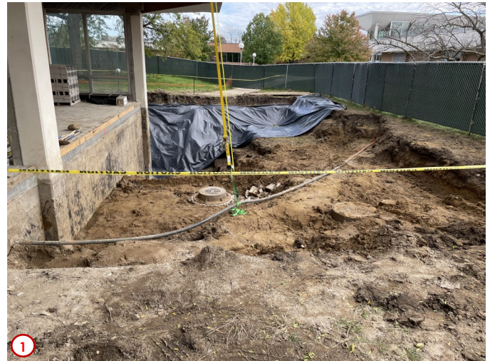
Photo #1 shows the progress of the excavation around the southern perimeter of the basement. Despite the heavy rains earlier in the week the contractors were still able to complete the work needed on the east face to expose the basement walls for waterproofing. Additionally, the existing utility vault was exposed and lowered. As more excavation is done the vault will be lowered more and then finally abandoned and grouted solid as, again, it is no longer needed.
