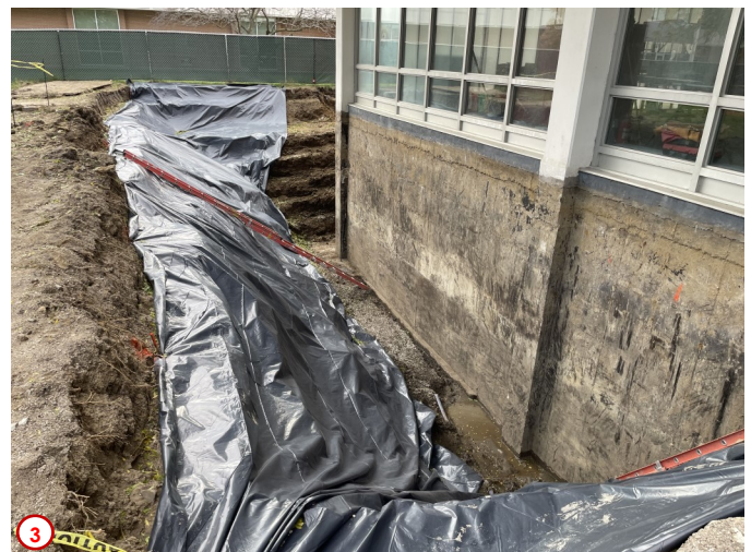
Photo #2 was taken on the east side of basement and shows the entirety of the wall surface exposed that will eventually receive the waterproofing treatment. The treatment will be done in stages and similar to how the excavation is being carried out in layers the installation and backfilling will happen in parts as well. This will happen for two reasons: 1) to be able to control the installation so as to work in smaller and more manageable sections, and 2) to allow for proper compaction of the backfill as it is being placed.
