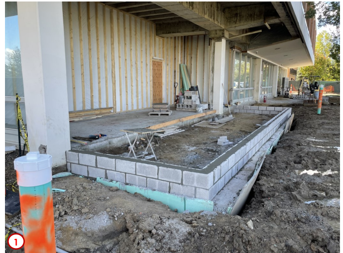
Photo #1 shows the now completed foundation system for the addition off of the northwest corner of the first floor. Next week the contractors will fill in the depressed area between the foundation and existing walls with compacted stone and place the new concrete floor slab on top of the fill. After the new floor slab has time to properly cure the new curtain wall system can start being installed in an effort to weather-proof this portion of the first floor.
