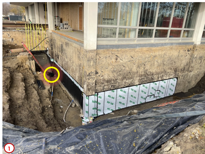
Photo #1 was taken earlier in the week and shows the work being done to waterproof the basement walls and backfill to make way for the future addition in this area. Highlighted for you is the new drain tile that is being placed adjacent to the footing. The previous version of this tile was installed incorrectly at the wrong depth and therefore was ineffective. This is just one of the many legacy items that are being corrected with this project.
