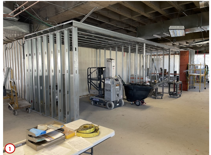
Photo #1 shows the progress of the installation of the rough wall framing for the new huddle rooms along the south wall of the Library. Two of these huddle rooms will be enclosed with glass and the other will be open. The two enclosed rooms will also have technology in them that will include flat-screen tv's that the students can connect to with their own devices.
