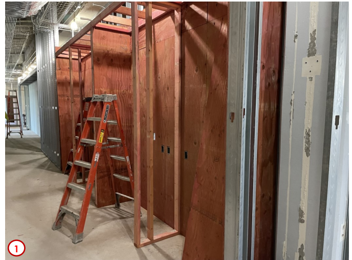
Photo #1 was taken in the new north corridor and shows the progress of the installation of the framing that will eventually house some private single occupant study booths for the students.
