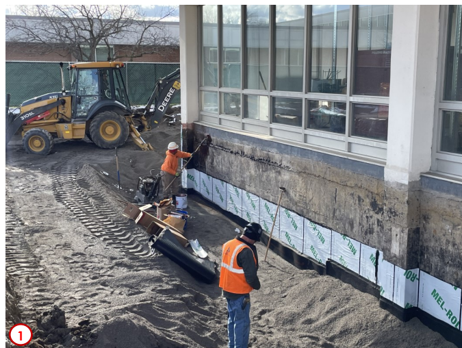
Photo #1 shows more of the installation of the waterproofing at the southeast corner of the building. This area is nearing completion, and is being backfilled with a better mix of soil and/or stone that will drain better than the original heavy clay that was originally in place.
