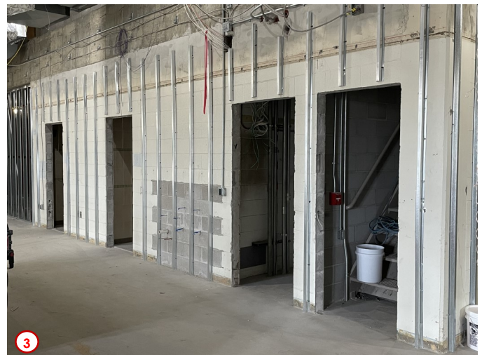
Photo #4 highlights the aforementioned fire sprinkler lines now installed in the future H/SS Office Suite (the black piping). The whole building will be fully fire sprinklered as per the new building code regulations, and will be yet another layer of new and/or improved fire safety systems that will help protect the staff and students that will be in this building once it opens for classes in the Fall of 2022.
