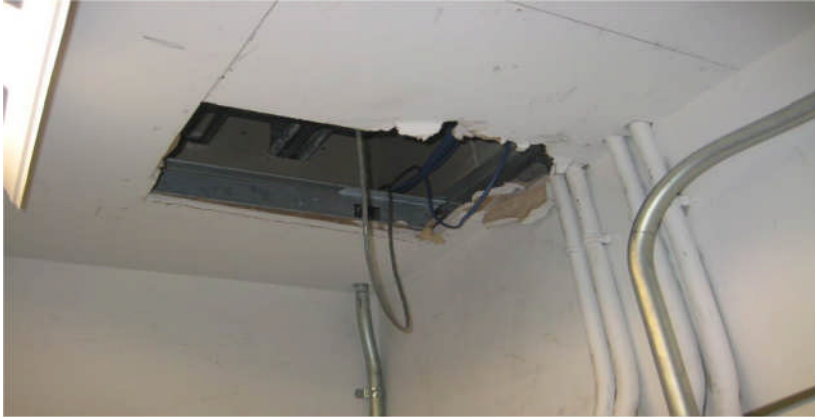
Whitman Center – breach in fire-rated ceiling assembly.
