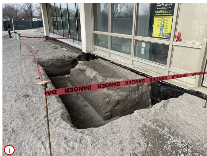
Photo #1 shows the excavation for the foundation system for the future screen wall that will enclose the area for the condensing units for the mini-split cooling systems in the main server in the basement. The foundation wall for this area will be placed next week along with several other miscellaneous areas around the south and west sides of the building.
