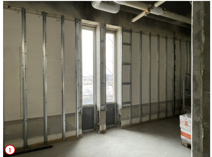
Photo #1 shows some additional demolition that happened this past week. Here the block wall from the window sill down to the floor slab was removed so that the entirety of the window frame is exposed. This was done because the new windows in the 2nd floor commons area only will be floor to ceiling which will allow for even more natural light into the interior of the building.
