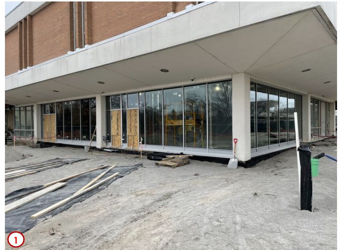
Photo #1 shows the progress of the installation of the new curtain wall system on the first floor. This past week an additional bay was completed and as seen in the photo is the left most bay which is near the west stair tower.
