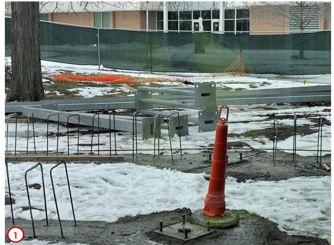
Photo #1 shows some of structural steel on site for the east canopy. Next week the contractors will focus on starting the process of erecting the frame for the east canopy, and once completed the finished canopy can begin.
