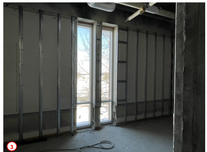
Photo #4 highlights the contractors working on replacing more of the existing window units along the southern face of the second floor. There are only three remaining sections to replace and then the entire second floor will be finished, and then the glazers will move back to the first floor and work towards finishing all of the remaining sections of curtain wall.
