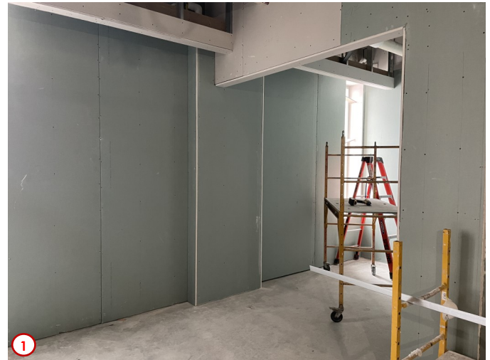
Photo #1 highlights some of the work happening in the future Writing Center on the second floor. The bump out in the background is where some framing and wallboard are now concealing some new hydronic piping that was installed that will support some radiant heating panels that will line the perimeter of the building and provide supplemental heating to ensure building occupant comfort.
