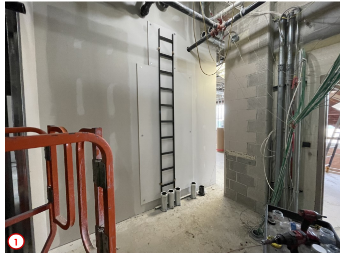
Photo #1 shows the progress of the installation of the new infrastructure needed to run data lines to and from the server room in the basement up through the first floor and then eventually onto the second in the new Electrical Room/Janitorial Closet. Here you can see the new penetrations from the basement and ladder rack that will help car-convey the new data lines being installed.
