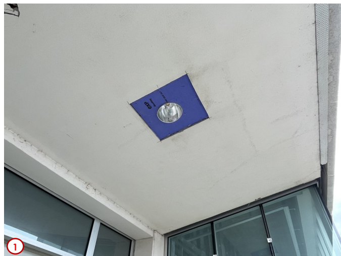
Photo #1 highlights one of the many instances where an existing can downlight has been removed in the building soffit and replaced with a new energy-efficient LED alternative. The process is quite labor intensive and involves installing new treated backboard, new stucco to match, skim-coating the whole soffit and then painting for a smooth finish free of any indications of new work.
