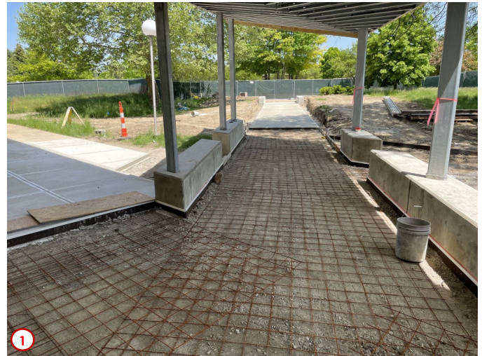
Photo #1 was taken looking out from the new east entry on the first floor looking towards the interior campus mall. Here one can see a portion of the concrete already placed for the new connecting side-walk and the balance of the area prepped so the remaining portion can be finished next week.
