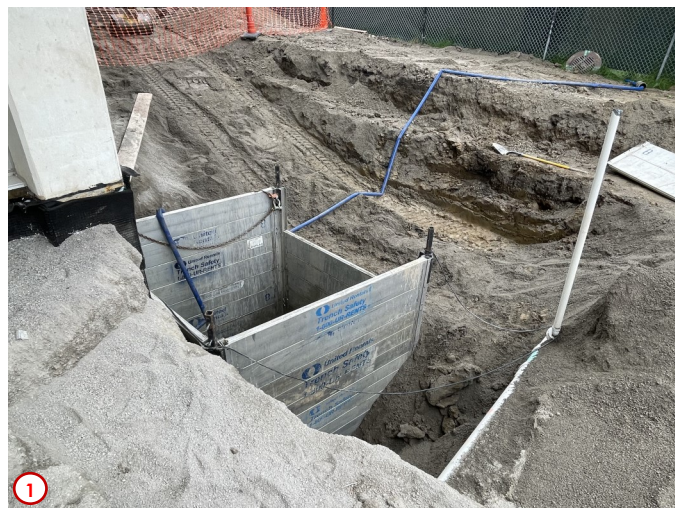
Photo #1 highlights the progress of the installation of the new storm water drainage structure outside the southwest corner of the building. In the photo one can see the shoring in place that holds back the surrounding soil to allow the contractors to set the structure in place and connect to the surrounding drainage lines. When this structure is finished this will allow the contractors to finish grading around the building and install the new sidewalks along the south side that connect the interior of campus to Parking Lot 7.
