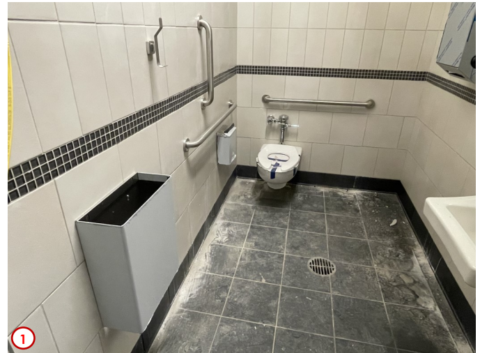
Photo #1 shows some of the remaining finish items now installed in the new unisex restroom on the second floor. Here one can see the accessories for the room have been installed including the wall mounted grab bars for the toilet, the trash receptacle, etc. Now this room is ready except for a good deep cleaning which will happen towards the end of the project just prior to occupancy.
