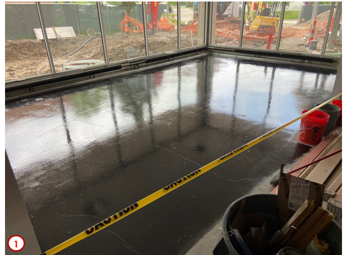
Photo #1 shows the completed installation of the epoxy floor sealer in the new student commons area near the new west entry. This sealer will eventually be covered by the carpet tiles that will be installed after it properly cures. This sealer is a safeguard as part of the space is over top of the main server room in the basement and was installed to help prevent moisture from this area possibly migrating through the floor slab and onto the electronic equipment below.
