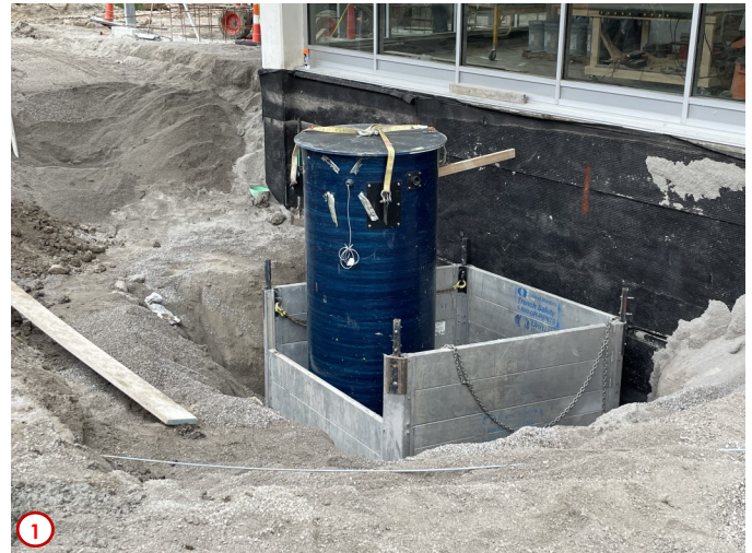
Photo # 1 shows the now installed drainage structure for the storm water system in this area. The contractors will now focus on backfilling around it and place the concrete collar on it which helps provide ballast and prevent hydraulic uplift. With this structure in place and back-filled the sidewalks in this area can be installed, as well finish grading. This will allow other items such as the finish landscaping to be installed as this project wraps up.
