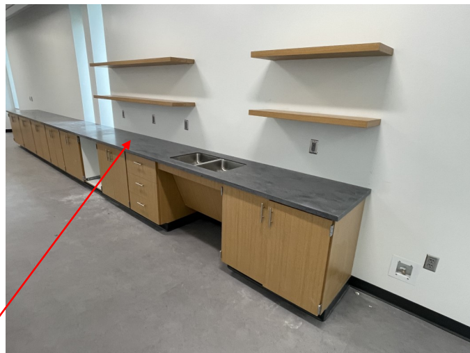
The top-right photo features one of the many countertops now being installed throughout the building. The one featured in this photo is located in the staff lounge in the H/SS Division Office Suite on the 2nd floor.
