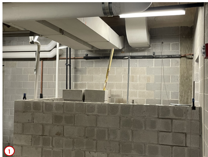
Photo #1 was taken earlier in the week and shows the block walls nearly complete. In the background you can see some of the plumbing infrastructure in place for the future mop sink that will be placed in the Janitor's Closet.
