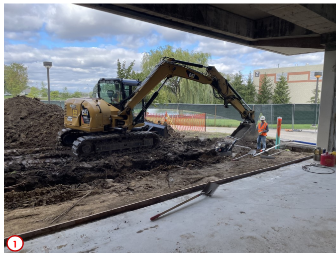
Photo #1 is of the excavation contractors backfilling after removing the old storm sewer line that was in this area. The previous line was located in the area of the foundation system for the planned addition on the northwest corner of the building and had to be removed. As mentioned in last week's report the new rerouted line is already in place and functioning well.
