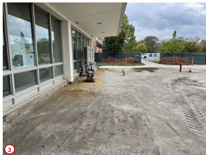
Photo #4 was taken at the southwest corner of the building and shows some site cleanup that was necessary for the targeted basement waterproofing to take place next week. The temporary scaffolding that was erected to convey building materials to the second floor has been taken down as well for now.
