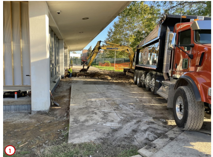
Photo #1 was taken early in the week outside the southeast corner of the CLRC and shows the very beginning of the excavation needed in order to complete the targeted waterproofing of the exterior face of the basement walls.
