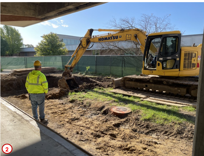
Photo #3 highlights the progress of the excavation on the east side of the building in the effort to expose the basement wall. This area is outside of the Little Theater and Classroom C-17. The basement wall will be scraped clean and then power washed. After that an adhesive will be applied which will help the new drainboard remain adhered to the wall. Finally, before backfilling a drain tile will be installed that will help convey storm and groundwater over to the storm sewer basin located near the southwest corner of the building. Then eventually the water ends up metering out into Plum Creek on the south end of campus.
