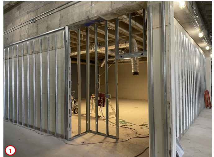
Photo #1 was taken near one of the classrooms on the second floor and shows some of the typical work being done there. At each of the classroom entrances the old entries were removed and new framing being installed to help further advance the efforts of making the building completely barrier-free and ADA compliant.
