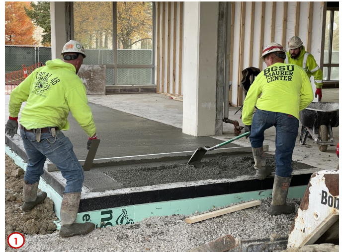
Photo #1 shows the contractors placing the concrete for the floor slab for the addition on the northwest corner of the first floor. This addition will house three new huddle rooms that will provide students with even more options as far as group study or socialization in the renovated Library.
