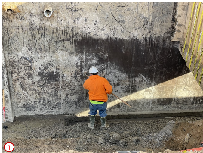
Photo #1 highlights the rather manually intensive process to prepare the surface of the basement walls to receive the waterproofing materials. The existing waterproofing materials have to be scraped off, and then the surface scrubbed so that it is clean in order to allow the new sealcoat and mastic for the drainage board to be properly secured.
