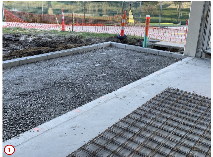
Photo #1 was taken earlier in the week and highlights the area of the addition to the northwest corner of the building and the now compacted fill in place. This fill will provide a solid base for the future concrete slab which will be installed in this area. In the foreground you can see the welded wire mesh reinforcing ready to be placed that will be imbedded in the future floor slab.
