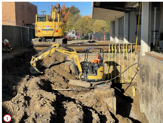
Photo #1 was taken earlier in the week as the excavation contractors are continuing the process of exposing the basement walls of the CLRC so that targeted waterproofing may happen. South of the CLRC there are a lot of underground items of concern such as the main fiber optic feed (the large black cable in the picture) and the steam tunnel running from HVAC Room 200 over to the CLRC. Added to all of this was exposing more of the existing storm water sewer system which meant the process of excavation took longer than usual in this area.
