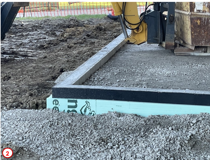
Photo #3 was taken later in the week after Photo #'s 1 and 2. Here you can see the vapor barrier has been installed over the compacted fill along with the wire reinforcing mesh. You can also see the dowel rods which will help provide stability between the new and existing slabs and help to create a uniform floor slab.
