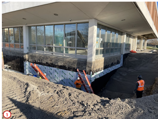
Photo #1 was taken earlier in the week as the contractors were finishing the targeted waterproofing on the west face of the basement wall. Here they are on the other side of the wall from Room C-17 which is where the main server room is for the campus. This waterproofing will help to provide yet another layer of protection to keep excess moisture out of that room and away from the very costly and sensitive equipment housed in that space.
