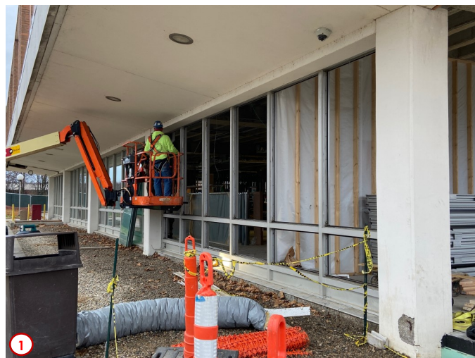
Photo #1 was taken earlier in the week and shows the glazing contractors installing some of the new curtain wall frames on the north side of the building. These new frame systems are thermally broken which means the exterior and interior faces are connected by an insulating gasket that helps prevent heat or cold transmitting via conduction. The old system was one piece which was not energy efficient.
