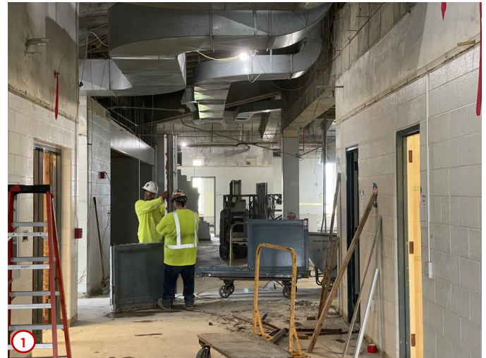
Photo #1 was taken last week when the remnants of the entrance and west walls of the LAL were being taken down. That area is now clear and part of it will become a new corridor, the rest will be part of the new Writing Center, and a classroom.
