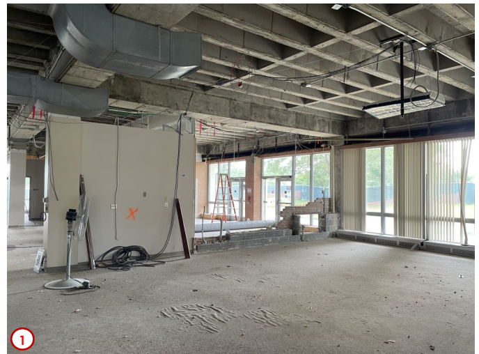
Photo #1 was taken over near the soon to be demoed library circulation desk looking towards the old entrance. As you can see the walls in that area have started coming down to make way for the new framing for the staff office suite and student conference room that will reside in that space.
