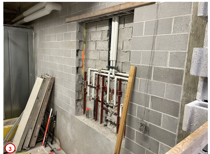
Photo #4 shows the progress of the construction for the new janitor's closet in the basement. Here one can see the new rough opening for the door into that space. The next phase will be for the contractors to tooth in new concrete block and install the new door and frame. However, this will not be finished until the new walls and floor slab are in for the closet.
