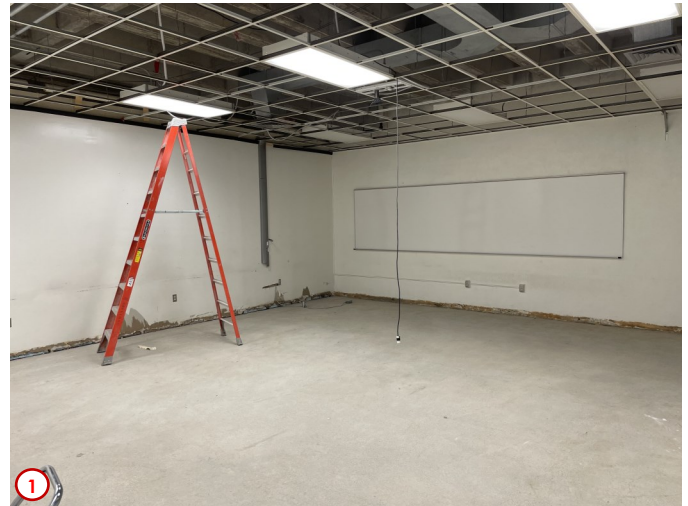
Photo #1 shows the progress of the typical demolition happening in all of the existing basement classrooms. You can see that all of the old tile has been abated and the mastic removed as well leaving a clean floor slab for the new carpet squares to be glued down at a later time. The existing ceiling tile and grid will be removed along with the lighting so that the new fire sprinkler lines can be installed along with the new ceiling and LED lighting.
