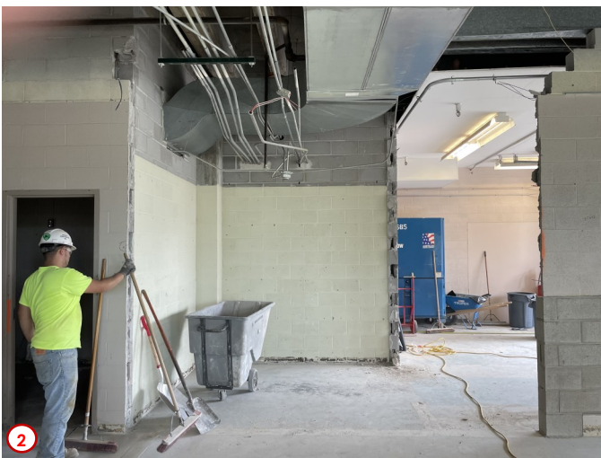
Photo #3 provides a glimpse into the demolition work being done to remove all the old walls that were part of the library staff offices, and reference collection area. One of the new additions will be connected onto that area which will house a classroom and computer lab. Additionally, part of that area will be the new main circulation corridor, the library main entrance, and part of the staff office suite. After all the walls are down the remaining carpeting will be pulled up, and then any existing mechanical and electrical infrastructure that needs to be removed to allow new construction to happen will be demoed as well.
