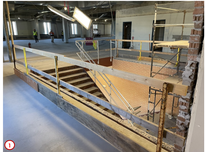
Photo #1 was taken in the area of the former office of the Dean of the Business Division and shows the now opened west stairwell on the second floor of the CLRC. Later this area will be where the contractors will be framing in the pocket where the fire curtain will be housed until needed.
