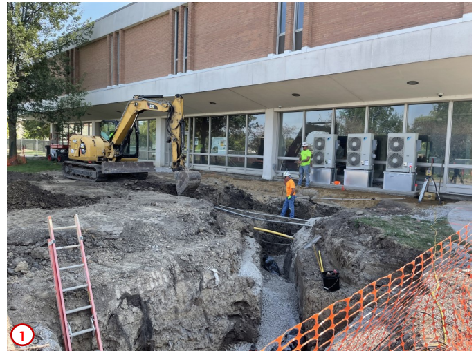
Photo #1 was taken outside the southwest corner of the building and shows the efforts of the excavation contractors to expose some of the existing utilities in the area and to prepare the site for new utilities that will help support the equipment and activities planned for the building interior.
