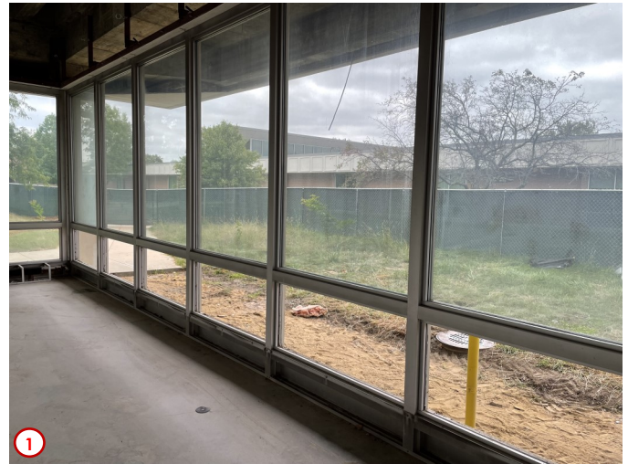
Photo #1 was taken just inside the southeast corner of the first floor of where the library offices were located. Here you can see that the contractors have started removing the glazing sections from the existing curtain wall system in preparation for removing the frames as work on the classroom and computer lab addition progresses.
