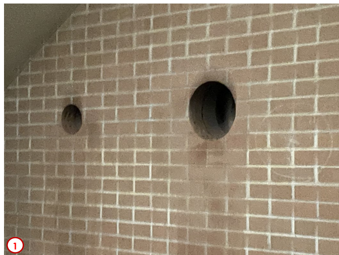
Photo #1 shows the completed bores for the new fire riser supply line and fire department connection in the new fire riser room in the basement under the west stair tower. The larger hole will be for the connection from the fire riser to the existing domestic water service loop on the west side of the building. The smaller hole will house the line feeding off the new fire riser to the fire department connection outside the building which allows them to hook up a truck to supplement the water in the building-wide fire sprinkler system.
