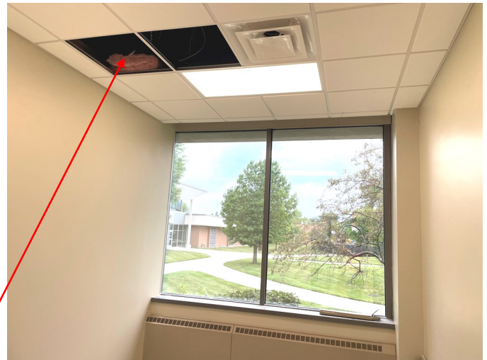
The top-right photo shows the ceiling being installed in one of the two private offices. For privacy reasons not only are the walls insulated but the ceilings as well.
