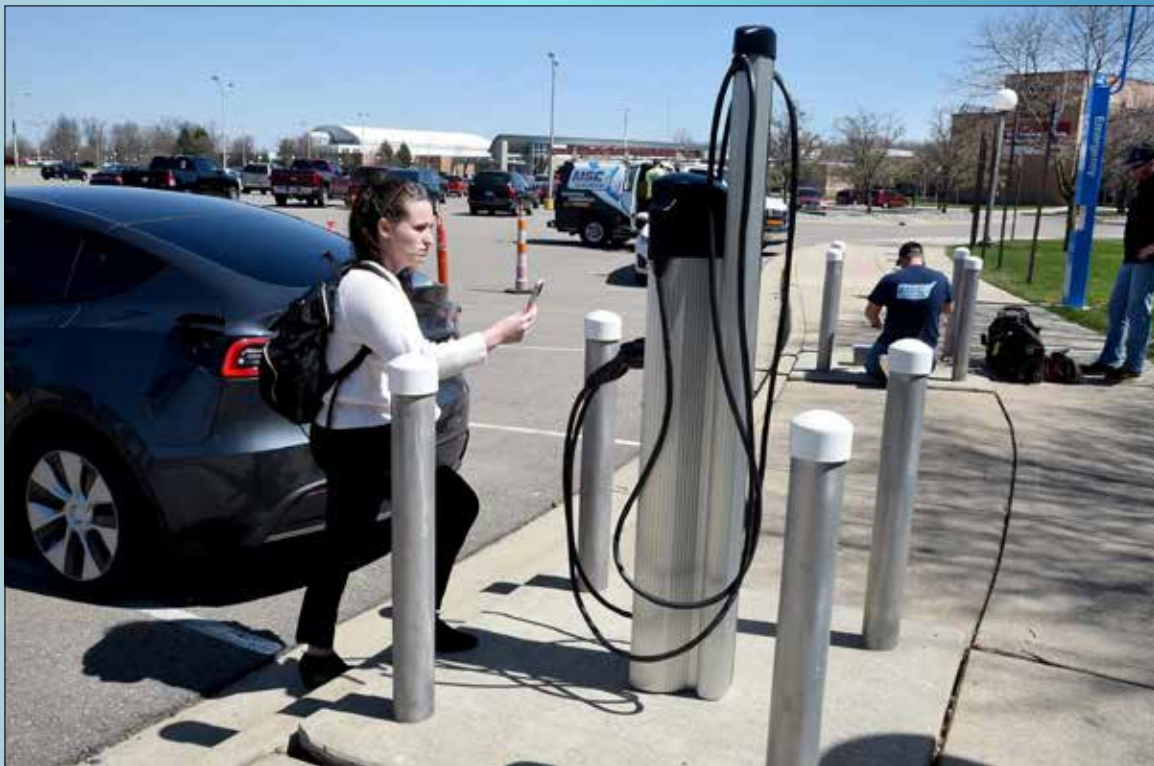
Katie Maller, Business Development Associate and Marketing Coordinator for EVUnited uses an app on her phone to connect her Tesla EV to the new EV charging station at Monroe County Community College in front of the La-Z-Boy Center/Meyer Theater. Electrical employees Troy Cox and Trevor VanHuyse, who set up the new EV charging station, cap the old charging stations installed back in 2017.
