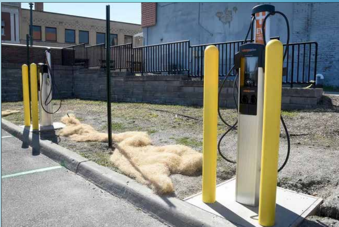
New EV charging stations are located at the east end of the Riverfront Parking Lot in Monroe nearest South Monroe Street and are accessible via the West Front Street entrances. (Both photos courtesy Tom Hawley/Monroe News)
