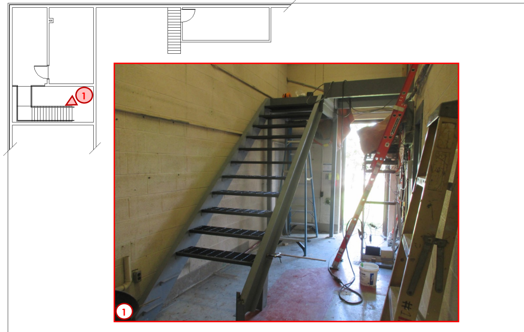
Photo #1 highlights the progress of the installation of the new metal stair case needed in the Physical Plan to access the renovated mezzanine area above the Locker Room that now houses the new IT Room. The old wood stairs were not code compliant and were not going to be functional enough to assist with access to the new IT Room and transporting equipment and allowing access for routine maintenance.
