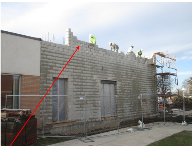
The top-left photo shows the progress of finishing the masonry shear wall on the north side of the addition. Now that the concrete roof slab is in place this work can be finished.
