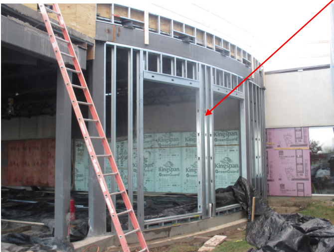
The bottom-left photo shows the light-gauge metal framing being installed for the exterior curved wall of the addition.
